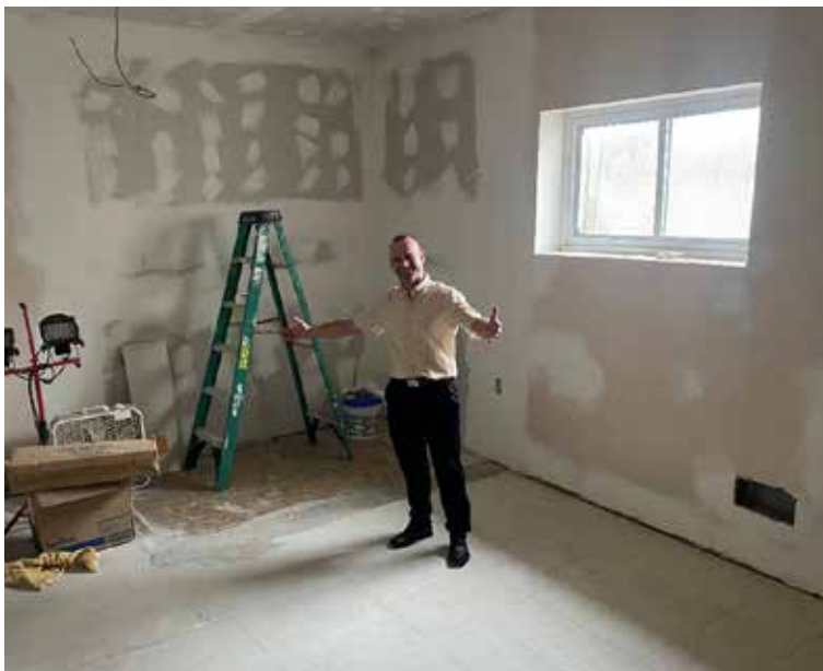
Fr. Bujdos assessing progress made on the renovation of a classroom at St. Michael's Church.
