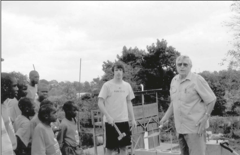
(L – R) Adam Check and his grandfather Dr. Thomas Check laying the ceremonial first layer of concrete block on a new addition of the St. John Bosco dormitory.
